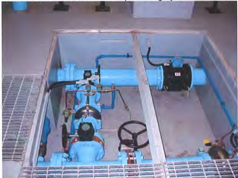
Figure 5 – Zone 4 Pump/Pressure Reducing Station on 30 th Street NE
