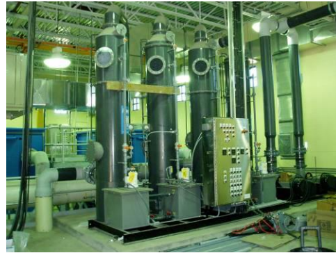
Train B Odour Scrubber
