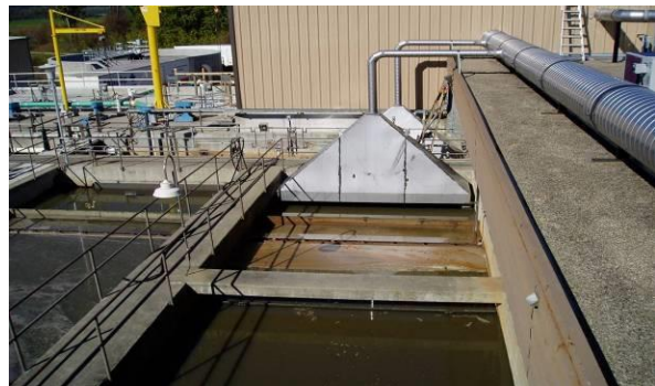
Primary Sedimentation Tanks
