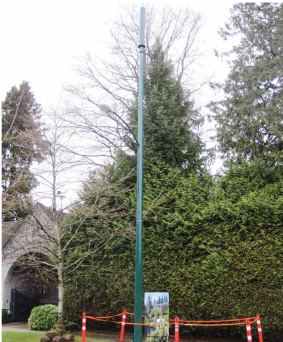
Example 1 of 13-metre tall streetlight antenna pole with connection cabinet at grade
