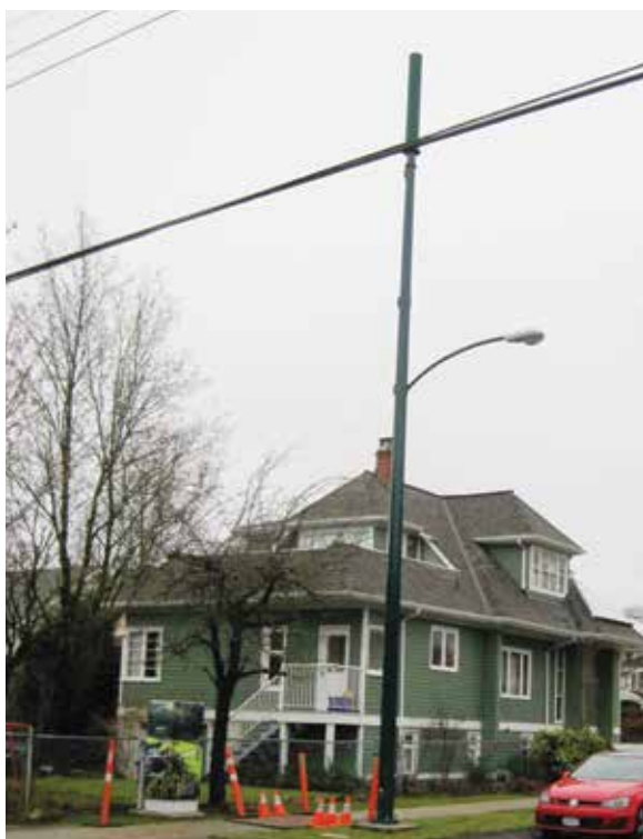
Example 2 of 13-metre tall streetlight antenna pole with cabinet.
