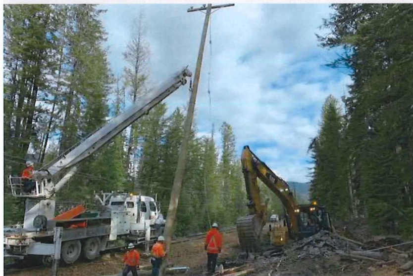
Crews near Field, B.C. working to restore power and protect the electrical supply for our customers. Photo courtesy of Jesse Winchester
