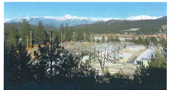
Located in Cranbrook's industrial area, Joseph Creek Substation is undergoing a $17 million upgrade. Photo courtesy of Sally Masters
