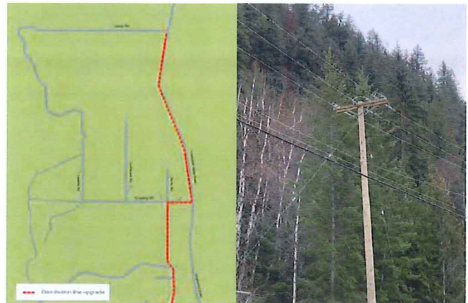
The old single-phase line was upgraded to a three-phase line. Photo courtesy of Curtis Head.
