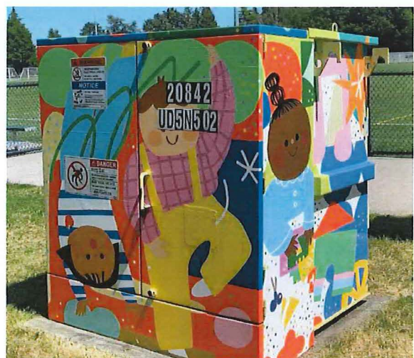
Example of a decorative wrap added to BC Hydro equipment. Photo courtesy of the City of Richmond.
