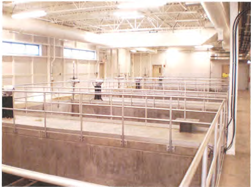
Figure 11 – Water Treatment Plant
