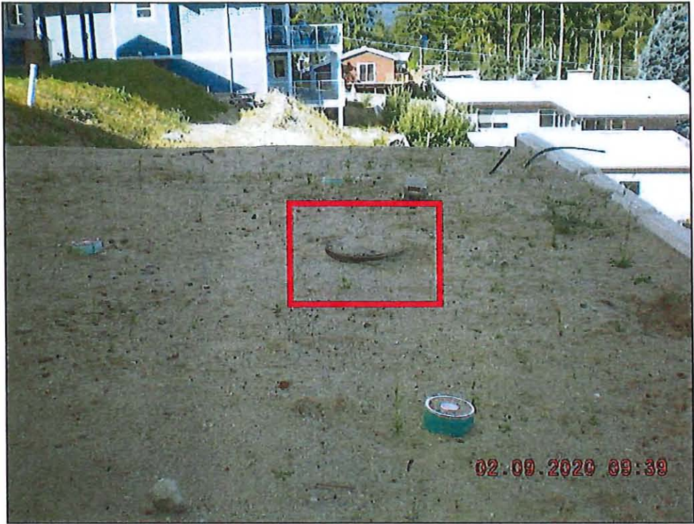
View of City sanitary sewer manhole in the statutory right of way.
