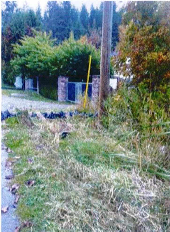
Sunday, September 30, 2018 - PICTURE #3 Unmaintained Drain and Culvert 210 11th Street, S.E.)
