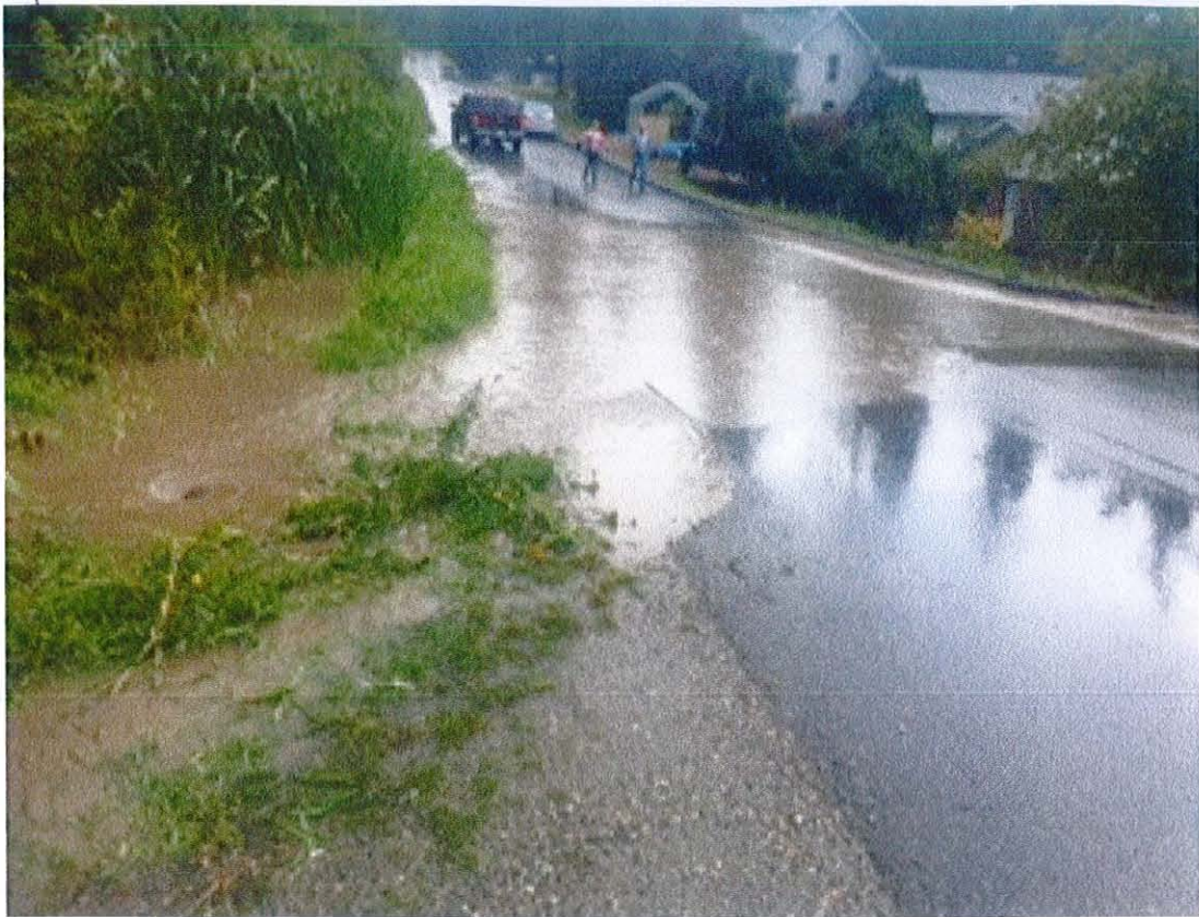
Sunday, September 16, 2018 - PICTURE #1 Storm Drain (after unplugged) in front of address 210 11th Street, S.E. Mike DeFelice and Reta Moerike in background
