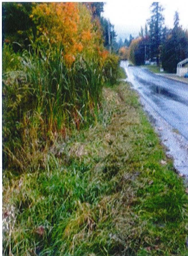
Sunday, September 30, 2018 - PICTURE #4 Unmaintained Culvert (210 11th Street, S.E.)
